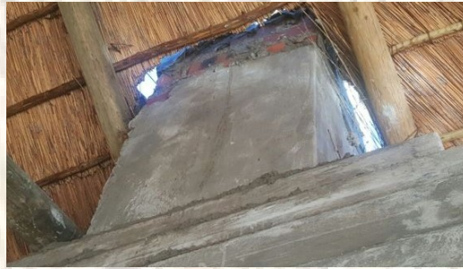
An opening cut through the thatch and a single brick wall built around the steel
