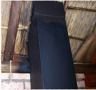
Thatch charcolize as a result of the heat from the steel
