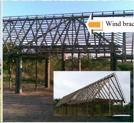
Show wind brace support beams bolted to the underside of rafter poles
