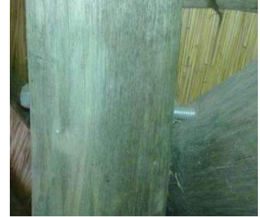
Incorrect positioning of threaded bar
