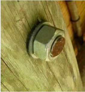
Incorrect washer size
