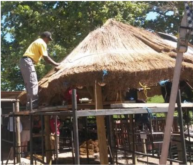
It was the first time in history that the TASA's Western Cape members built a roof together
