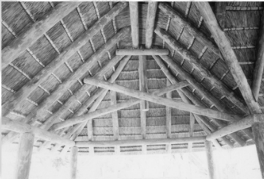
Photograph 11 Typical scissor-type truss configuration
